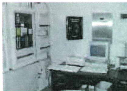
(Fig. 6.10) Fire command center with fire alarm and communications equipment, a work table, and adequate work space for the incident command staff.
