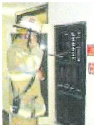
(Fig. 6.8a) Fire officer speaking into the handset at the control panel for a fire department communication system. This panel also houses the handsets used by firefighters at remote jacks.
