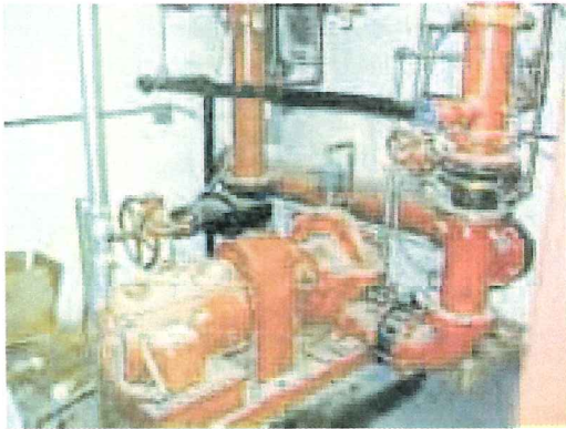
(Fig. 3.5) Fire pump.
