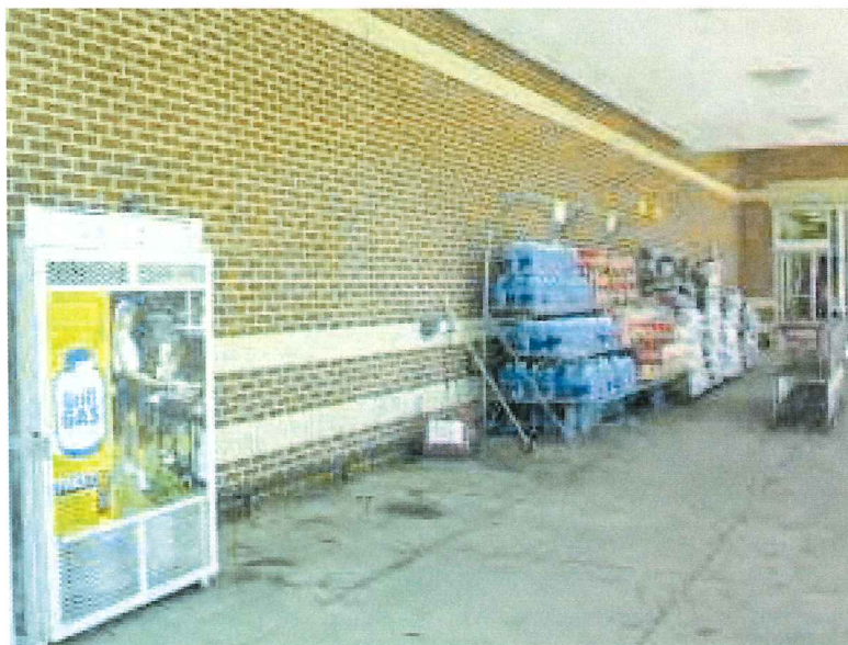
(Fig. 5.7) FDC in the cart area of a supermarket entryway. The FDC is located where merchandise or shopping carts could easily block it, or a fire in the adjacent propane storage area could restrict its use.
