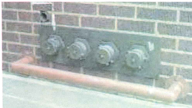
(Fig. 5.3) A 4-inlet FDC. It would probably be more efficient, and give the fire department more options, to have placed two, 2-inlet FDCs in different locations on this building.
