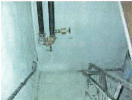
(Fig. 4.12) The feed for this standpipe was on a level above the fire department entry. The supply pipe was fed down (on the left) to the entry level, where the isolation valve was located. Then, the pipe was routed back upwards (on the right) to feed the standpipe riser.
