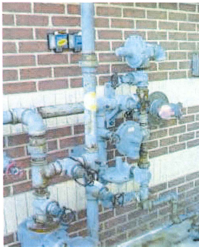
(Fig. 5.8) This FDC is located too close to the gas service and meter. The breakaway caps make it necessary for a firefighter to swing an axe or other tool to remove these caps. This is an accident waiting to happen that could be avoided through careful design coordination.
