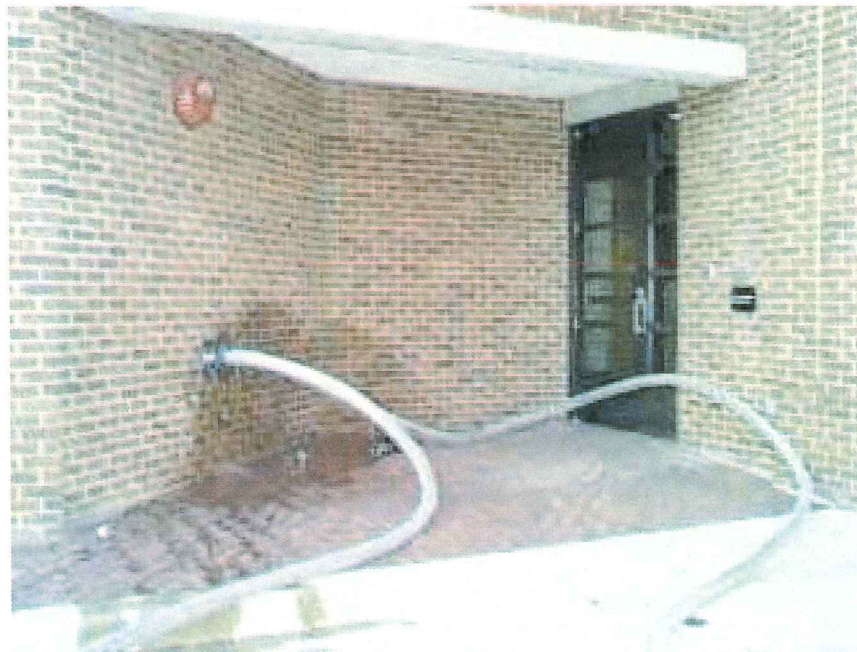
(Fig. 5.1) Charged hose lines connected to a wall-mounted FDC. The proximity of an FDC relative to building exits is discussed in the Location section at page 44.
