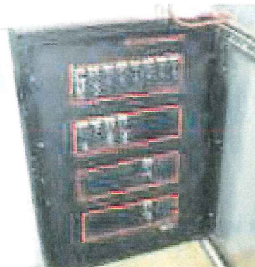
(Fig. 6.1b) Control panel.
