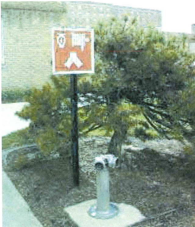
(Fig. 5.11) FDC sign with an NFPA 170 symbol for both sprinkler and standpipe systems.
